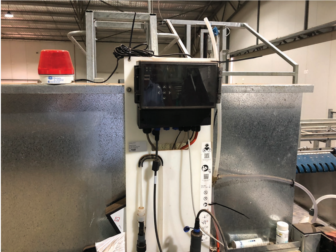
Figure 23. An automated monitoring and alarm system to manage sanitiser levels in a dump tank.
