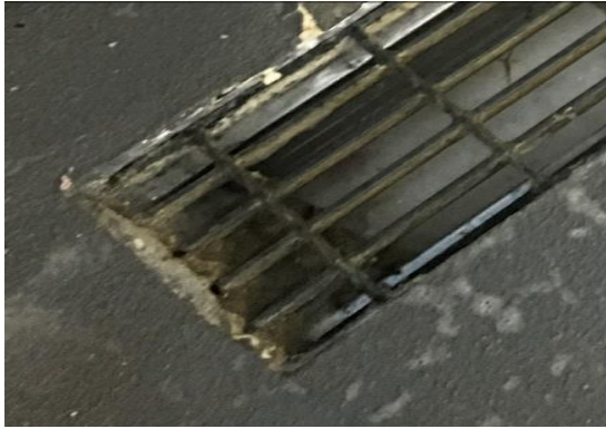
Photo B: trough drain grates were seized in place
